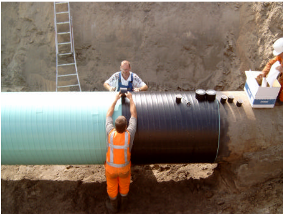
Figure 1. Protection of a gas transfer line with Stopaq wrapping band CZ H and PVC tape. (Green part: Stopaq wrapping band with outside PE layer; Black part: PVC coated tube).
