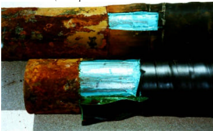
Figure 2. Released parts of coating after 7 years. (Metal parts are blanc: no corrosion could be observed)
